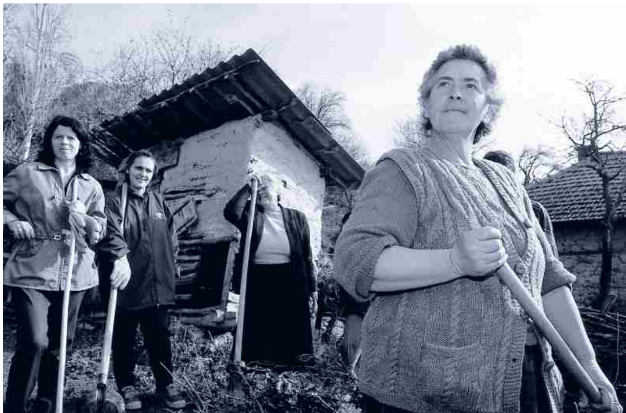
Small numbers of women in the CEE and CIS have found work in the construction trades. These women are building a drainage channel in Kosovo. Photo:Ky Chung/UNMIK/DPI
